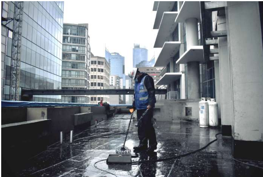
Above: An SMT Technician performs a Digiscan service on an inverted roof membrane
